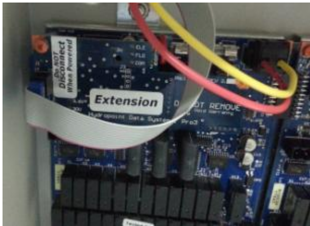
Figure 3. Power and Ribbon Cables Connection at Extension Chassis
